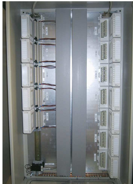
I/O cabinet with 12 units installed
